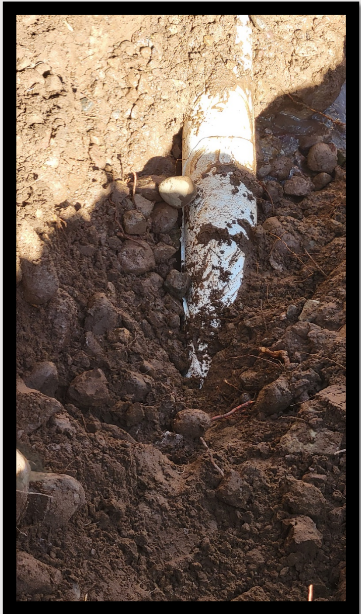
Crack in the water main on Baca Grant Way
