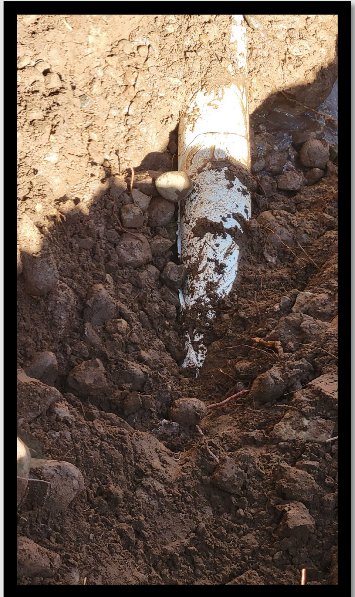
Crack in the water main on Baca Grant Way
